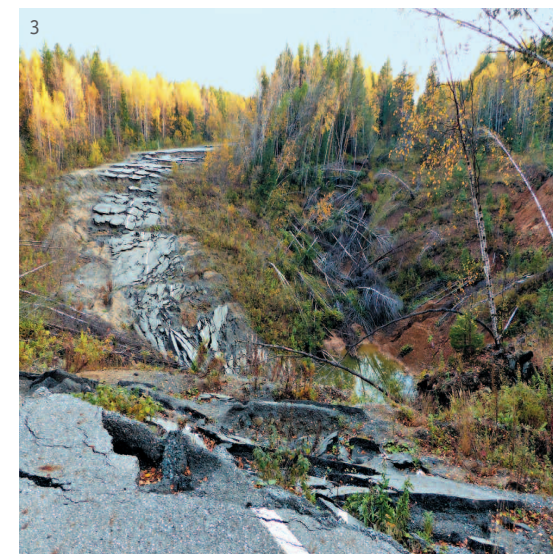
3. Pot-hole in the collapse zone of the Yuzhniy body, Severopeschanskaya mine.
